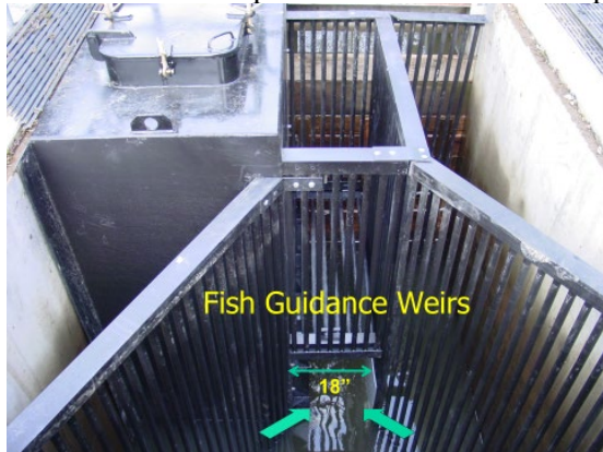
Upper Bennett Weirs and Vault (fish pass window and then exit to river)
